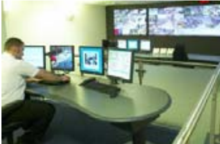
Operators using the GUI interface and central management system provided by Cortech Developments.
